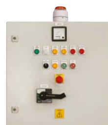
30kW Pump Control Panel
